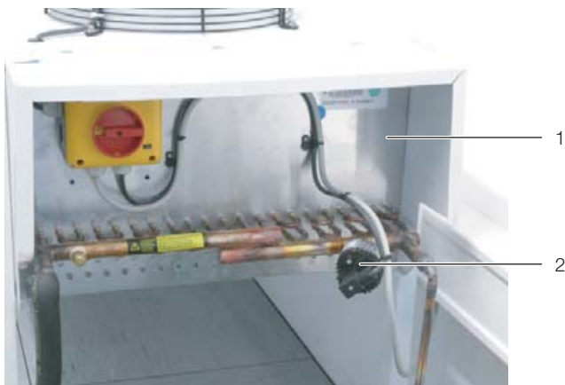
Fig. 31: Pressure switch on the condenser
