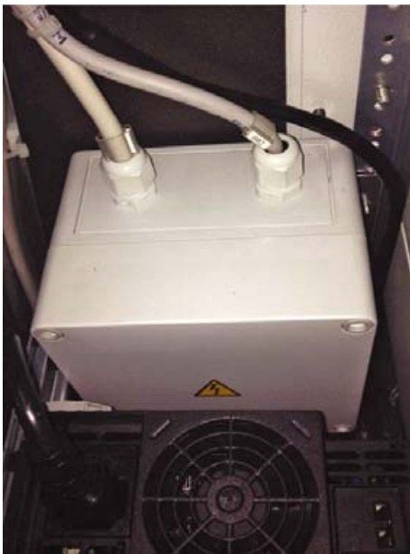
Fig. 54: Additional box for the thermal protection of the electrical heaters
