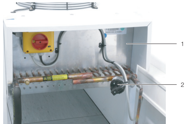
Fig. 29: Pressure switch on the condenser
