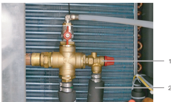
Fig. 27: Safety valve at rear
