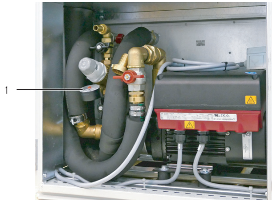
Fig. 48: Manometer in the water circuit
