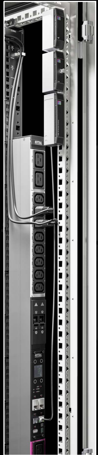
Application-specific sensors may be incorporated into the central monitoring system directly via the PDU's CAN bus interface.
