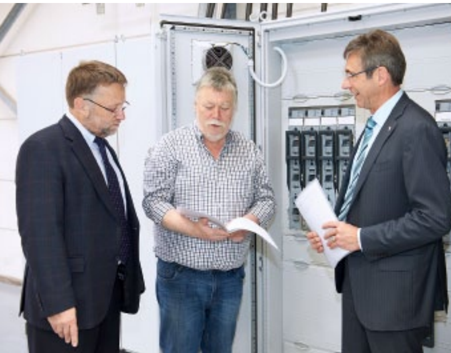
Wolfgang Ehmer (Rittal consultant), Mathias Krakrügge (a member of the energy technology team in Breckerfeld) and Uwe Braselmann (owner of deller plastics) with the ISV distribution enclosure system from Rittal, which is extremely easy to install.
