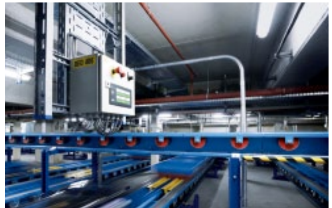
Securely housed in enclosure technology from Rittal – control technology belonging to the baggage handling system at Frankfurt Airport.
