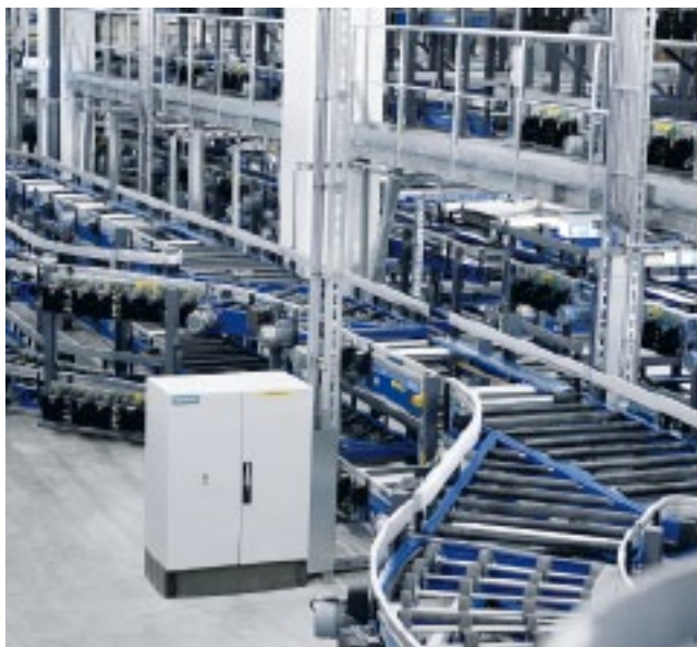
Decentralised CM compact system enclosures from Rittal offer reliable protection for Siemens control technology right in the middle of the baggage handling system.
