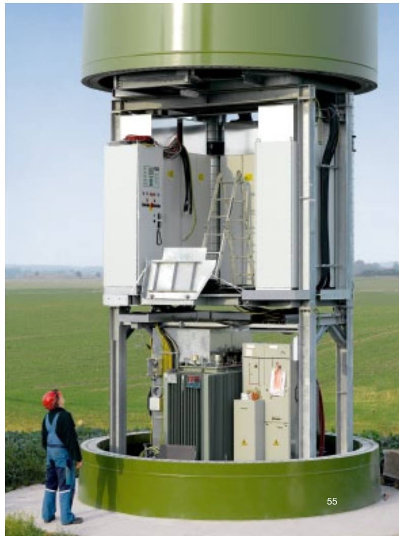
Enercon uses TS 8 enclosures from Rittal to house the frequency converters for its wind turbines.
