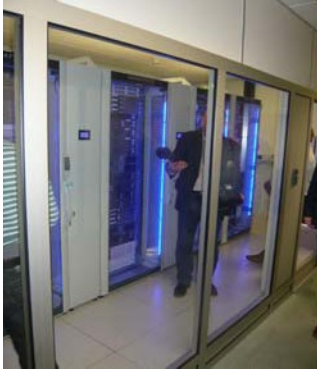
LCP plus in serverruimte
