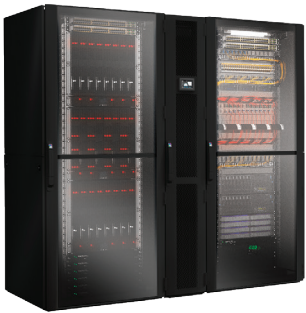
Data center row view
