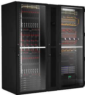
Data center row view
