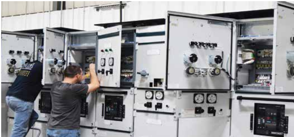
Rittal supplied a total of 114 TS 8 enclosures, including standard, modified and electromagnetically compatible models. These enclosure systems improve reliability, save energy, reduce emissions, lower maintenance costs, enhance safety and support maritime regulations. Since on-site modification was impossible, and scrap recycling of any modifications was unacceptable, the Rittal enclosures arrived ready-to-install.
