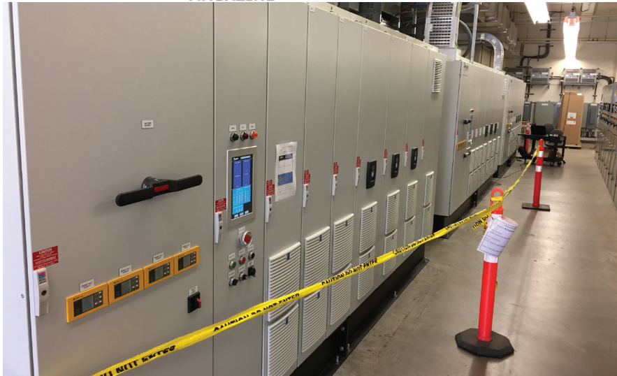
The enclosures had to contain all the critical equipment in a small area, while keeping the components environmentally safe and secure.
