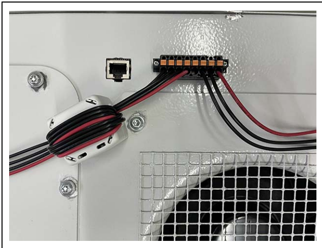
Fig. 10: Signal cable with mounted ferrite core
