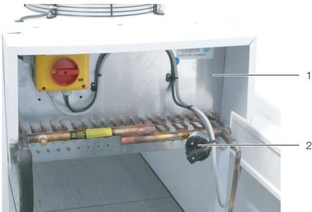
Fig. 25: Pressure switch on the condenser
