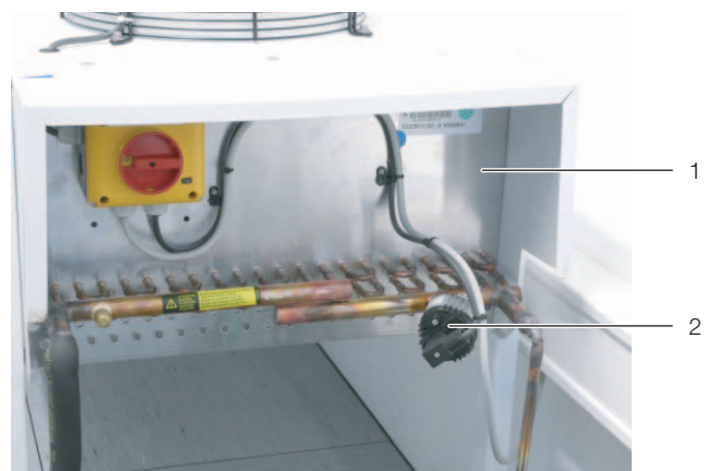
Fig. 27: Pressure switch on the condenser
