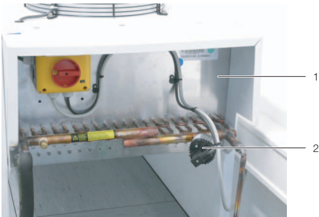
Fig. 27: Pressure switch on the condenser
