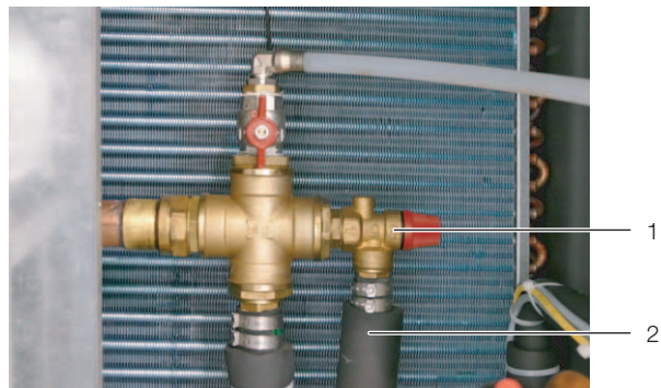
Fig. 24: Safety valve at rear
