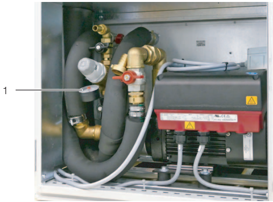
Fig. 44: Manometer in the water circuit
