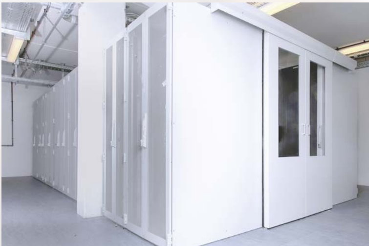
The Manner servers are accommodated in 14 Rittal TS IT racks, which are arranged in two rows facing one another to form the cold aisle.
