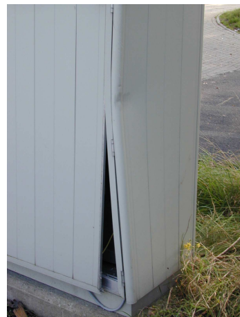
Image 1: Deformed enclosure after impact
