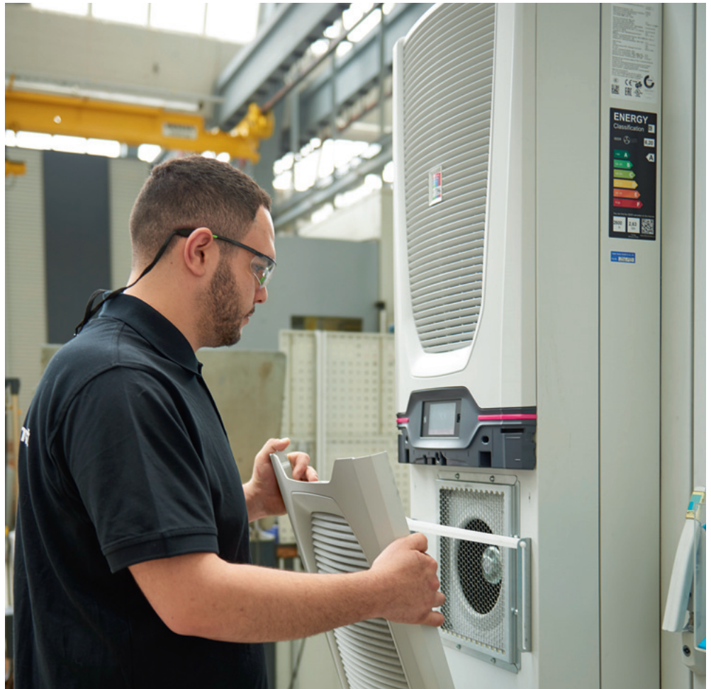
Figure 3: Retrofitted with savings: After the conversion to the new Blue e+ chiller generation, more than 70 percent or 25,000 euros per year in energy costs were saved.
