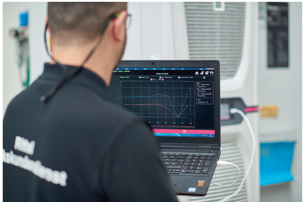
Figure 2: Everything in sight: An employee from the Rittal Manufacturer's Service checks the current efficiency values of the Rittal Blue e+ cooling units at Voith Turbo in Heidenheim.
