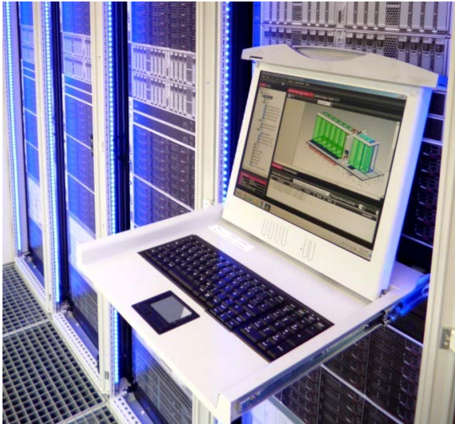
Figure 8: RiZone – RiMatrix S – Single6 installation
