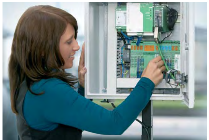
Reliable transmission of process data via GSM modems
