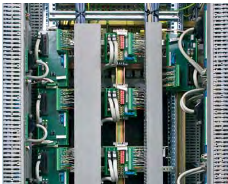
Interface modules with system cables to the control system
