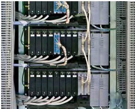
System cabling Yokogawa control system CS3000 R3
