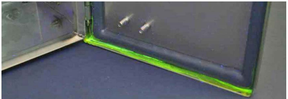
Figure 12: Not all the contamination is removed after a conventional enclosure is cleaned.
