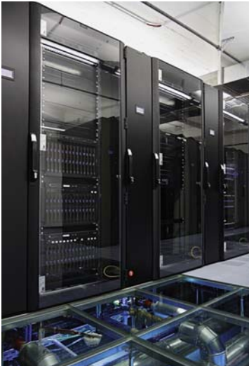
In an economically run data centre, all consumers are optimised for efficiency.
