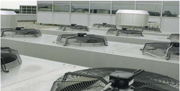
Low-energy free cooling has a number of uses.
